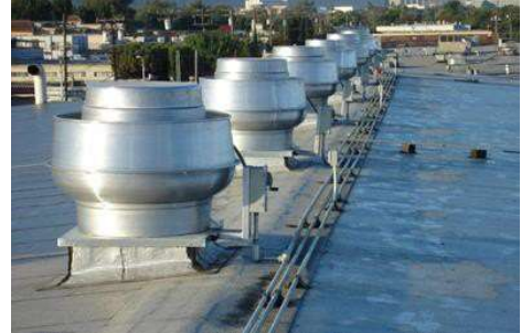
Explosion-proof exhaust fans for the first level of ventilation.
